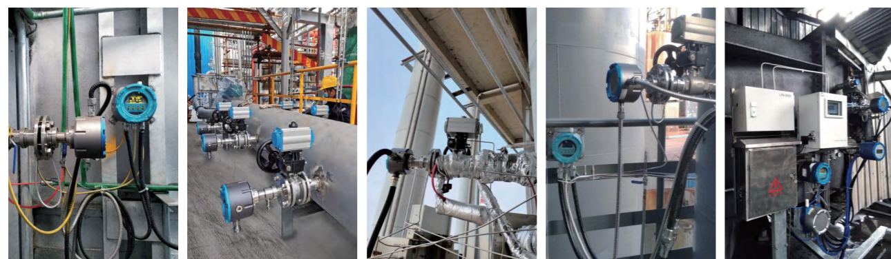
Furnace combustion optimization high temperature 1400°C
