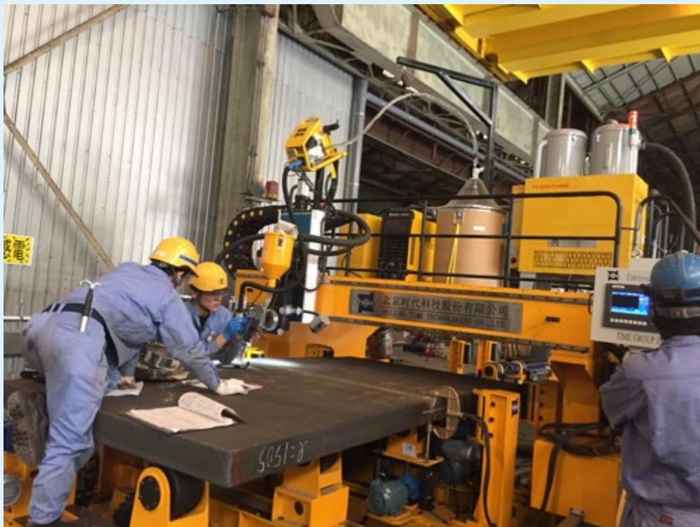
Narrow gap welding of stainless steel with ultra-high deposition rate (Exported to Japan)
